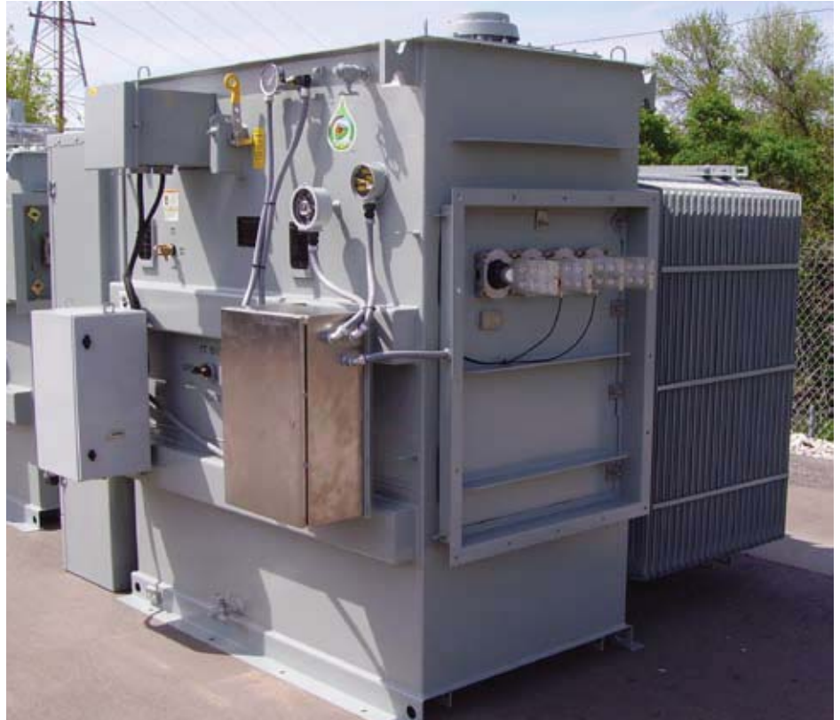
Figure 1. Unit type substation transformer equipped with low-voltage transition flange and high-voltage full height air terminal chamber.
